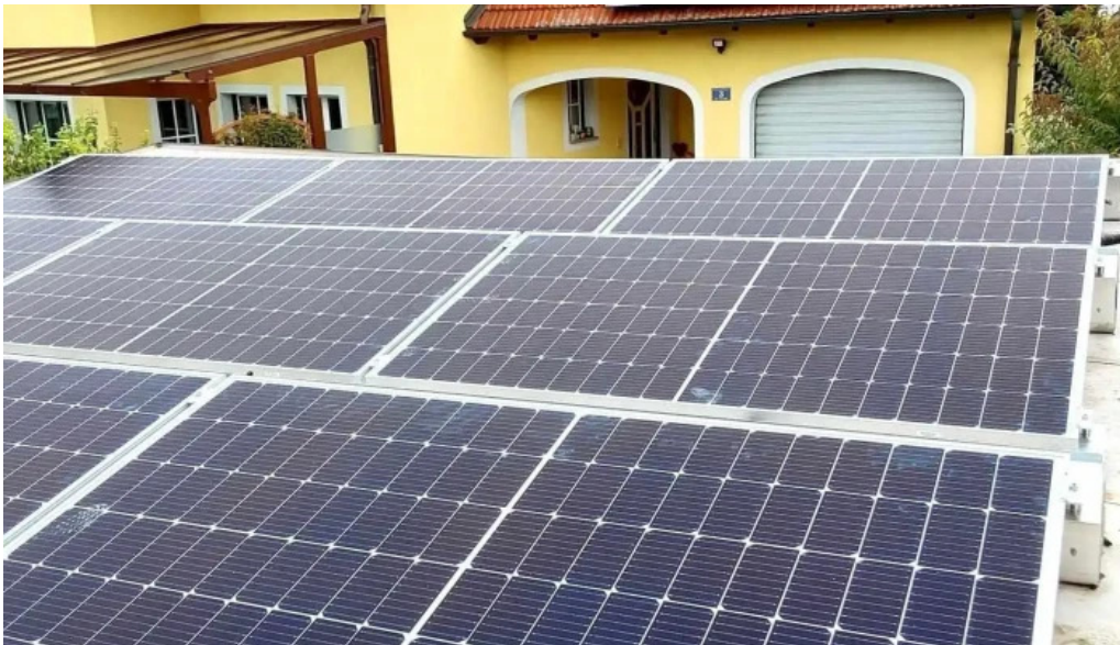
Harisberger fair energy photovoltaik stromspeicher alle
