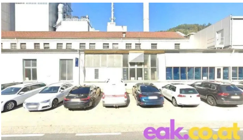
Be energised charging station st gertraud
