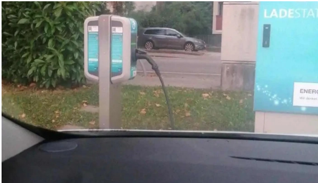
Energie ag oberosterreich charging station alle
