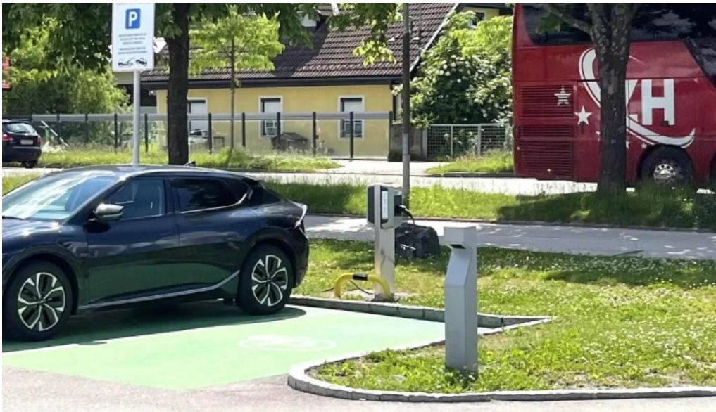
Hastobe charging station ladestation fur elektrofahrzeuge
